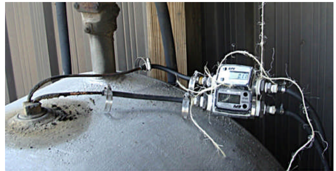
Figure 5 Flow meters and fuel tank providing fuel to compressor engine
